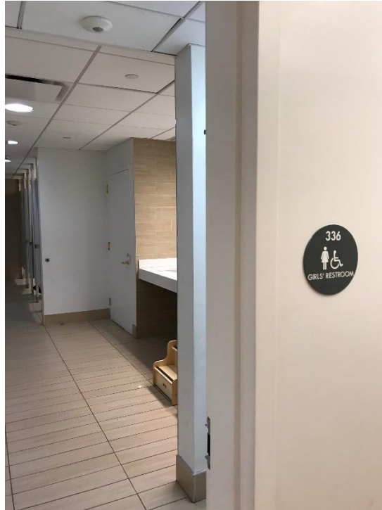
No privacy barrier, main door removed Other solutions include door to stalls removed, shared sinks in open area/corridor
